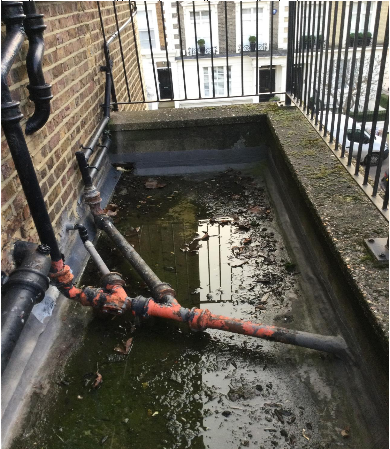
Existing flat roof with existing pipework, show fixing of the railings to parapet wall
